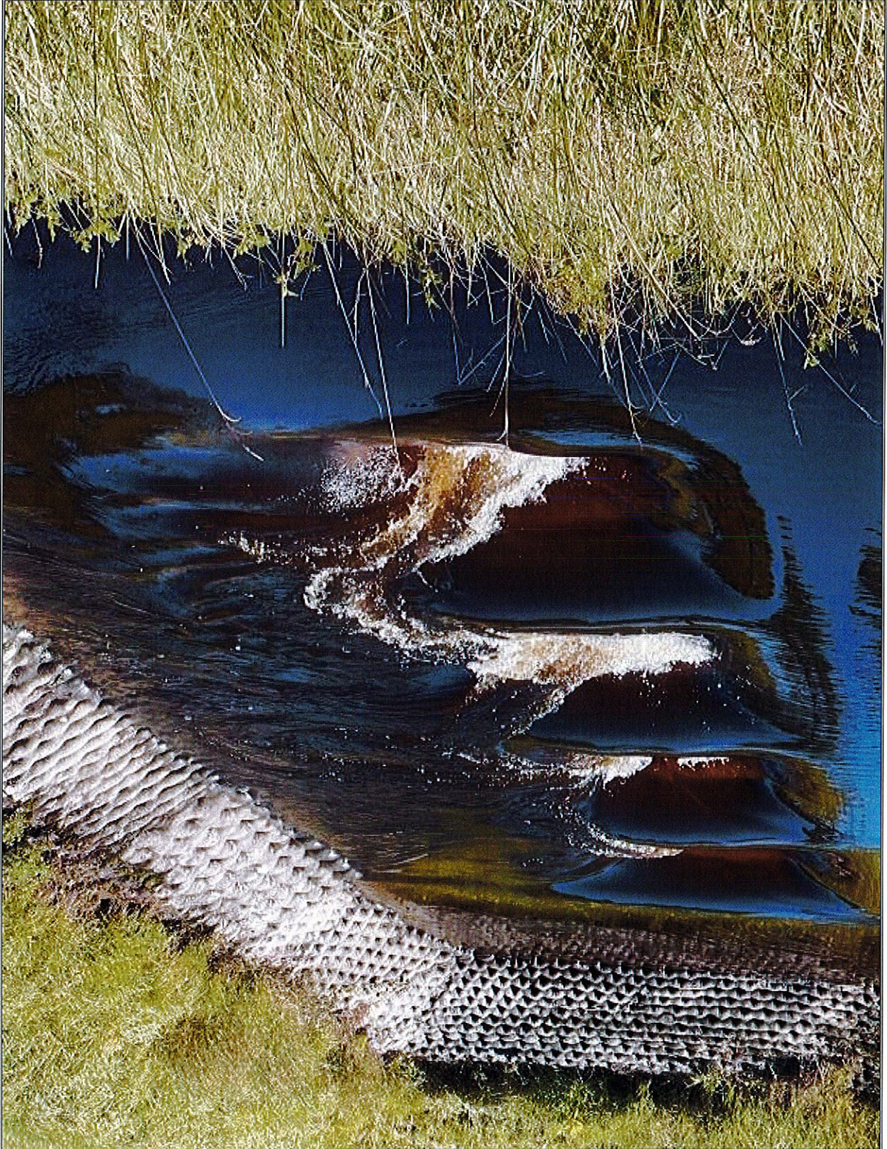
Canal 5 Anti Vortex Damage
